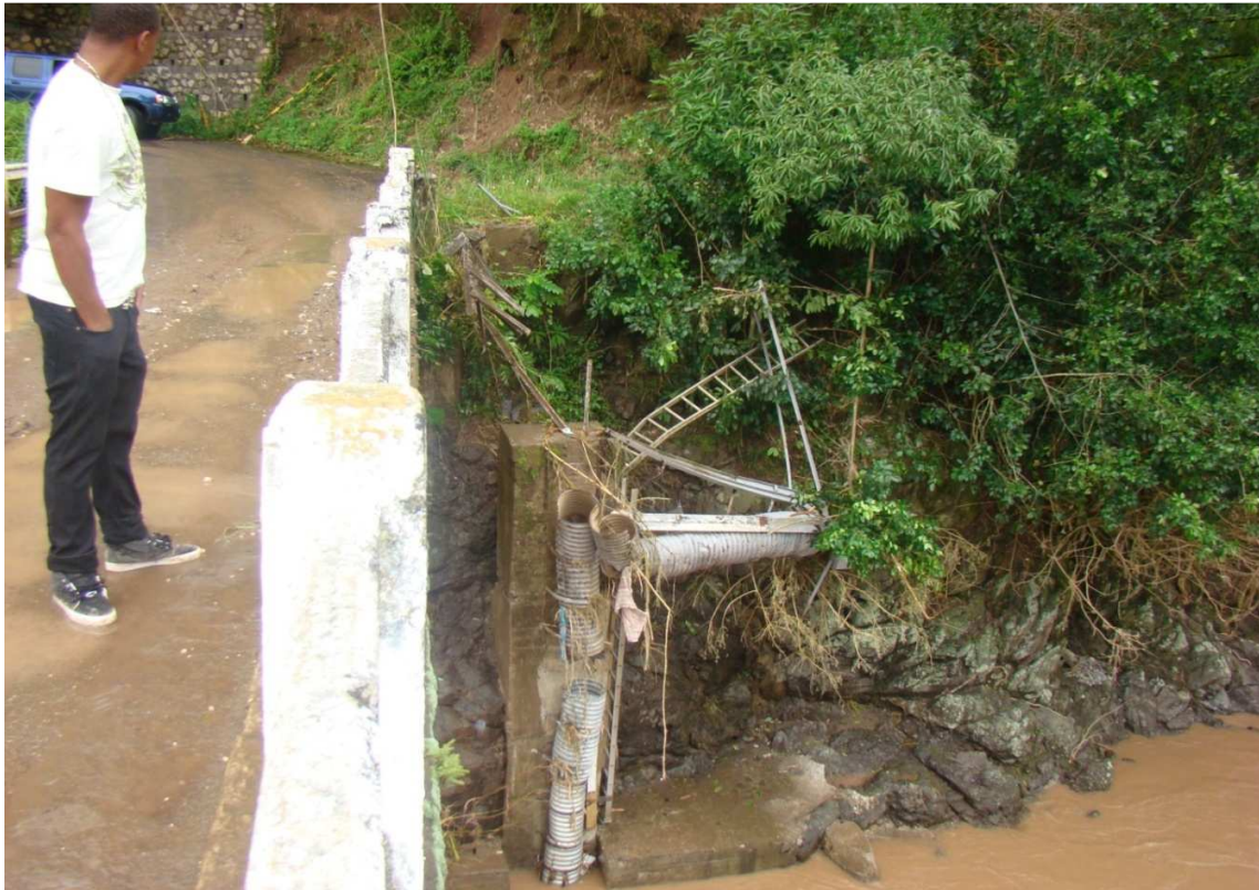
Photo 1: Damaged gauging station at Blakes Bridge on the Wag Water River in St. Mary
