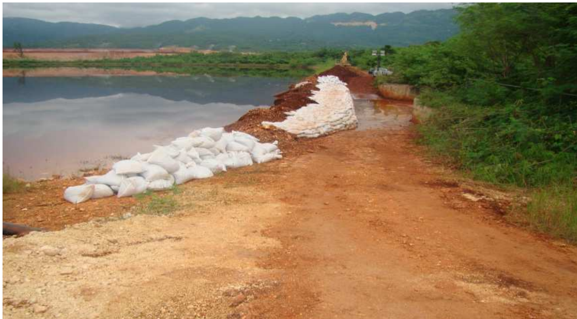
Caustic Effluent in the Holding Pond at Ewarton Works, Charlemont, St Catherine Exceeds its holding capacity and overflows via the spillway. Sand bags used to obstruct flow through the spillway. Photo taken October 2010
