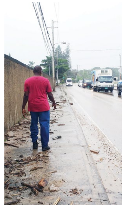
Concrete wall that runs along east-west alignment near the Runaway Bay Town Center (WRA Team member shown for height reference)
