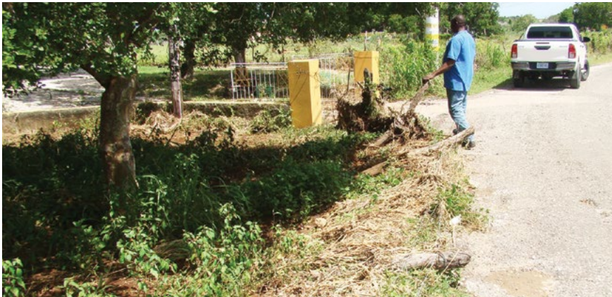
WRA team member assessing fence toppled over by flood waters in Treasure Beach, St. Elizabeth
