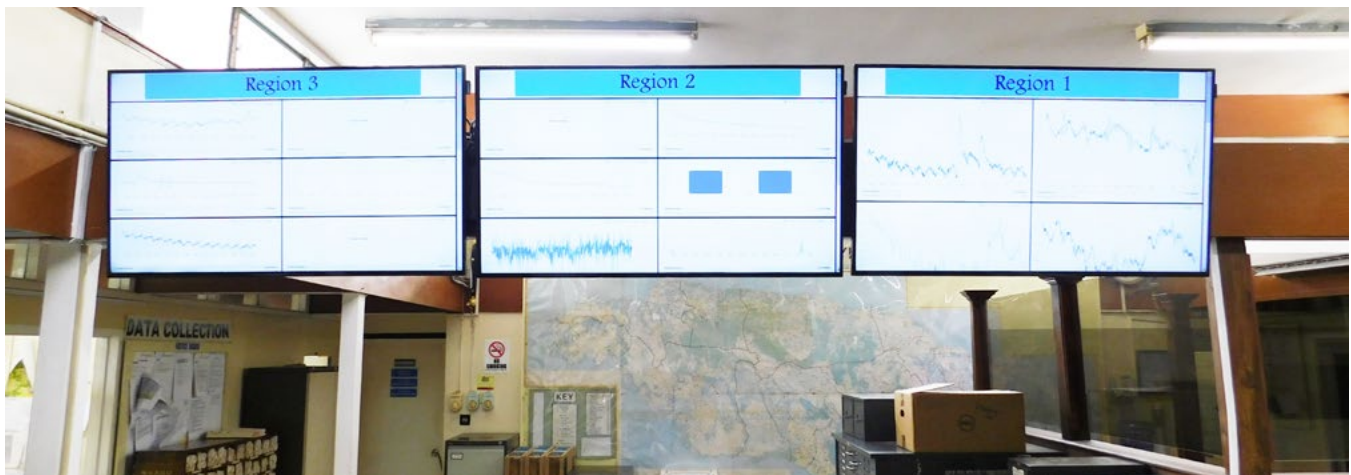
Figure 10: 48inch monitors from which stream flows are monitored.
